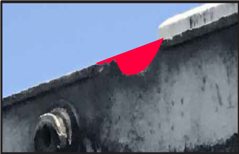
LOSS - loss of portions of marble due to general weathering and erosion
