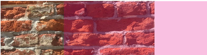
HEAVILY DETERIORATED BRICK
