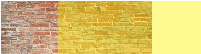
DAMAGED BRICK FROM STUCCO REMOVAL
