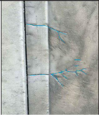
CRACKING - Narrow fissures in a block of masonry.
