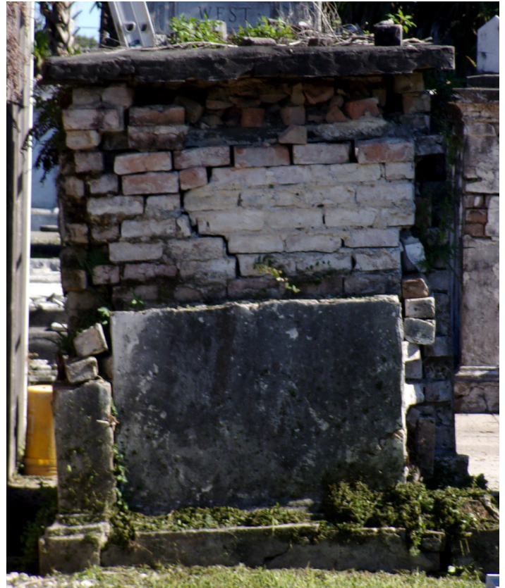
Figure 87. View of the rear of tomb shown to the left; partially missing stone veneer and bricks, vegetation.
