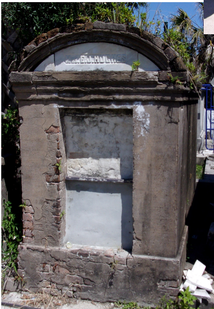
Figure 83 (to the left). Missing closure tablet, significant biological growth, missing stucco exterior and loss of some bricks on the parapet.
