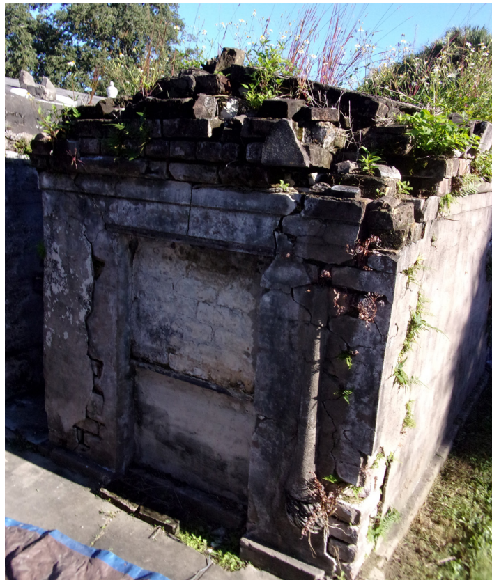
Figure 88. Severe vegetation and cracking, missing features (enclosure tablet and inverted torch), missing bricks and stucco.
