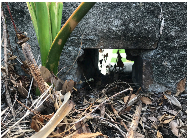
Figure 19. Photograph showing the brick that was removed on the southwest wall of the Teutonia Lodge in an attempt to create a draining system.
