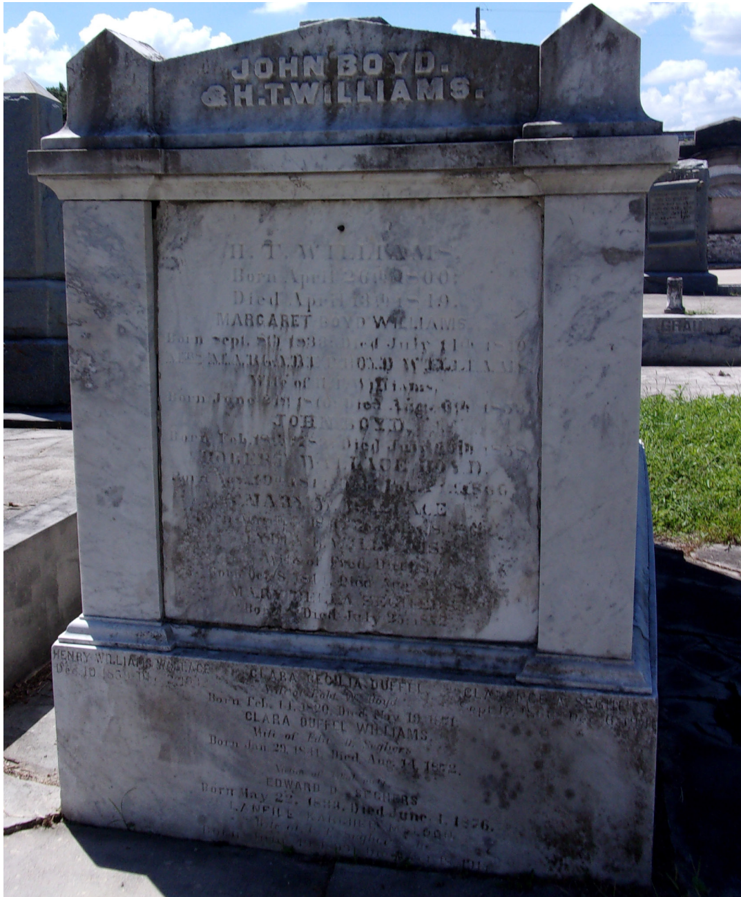
Figure 72. Structurally sound family tomb, showing mainly cosmetic issues (staining), which are relatively easy to repair. Marble is in good condition.
