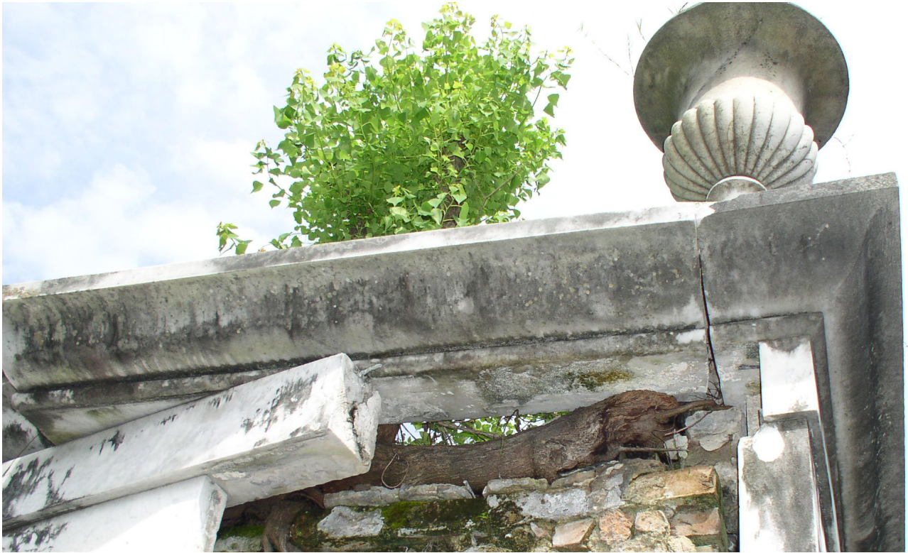
Figure 21. Photograph showing a tree and roots growing out of the northwestern wall/western corner of Teutonia Lodge, pre-stabilization efforts. Taken by Michael Duplantier, Sr., 2015.
