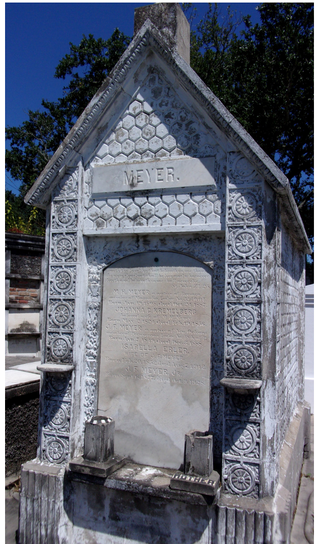
Figure 79 (to the right). Highly decorated, structurally sound tomb showing lots of staining.
