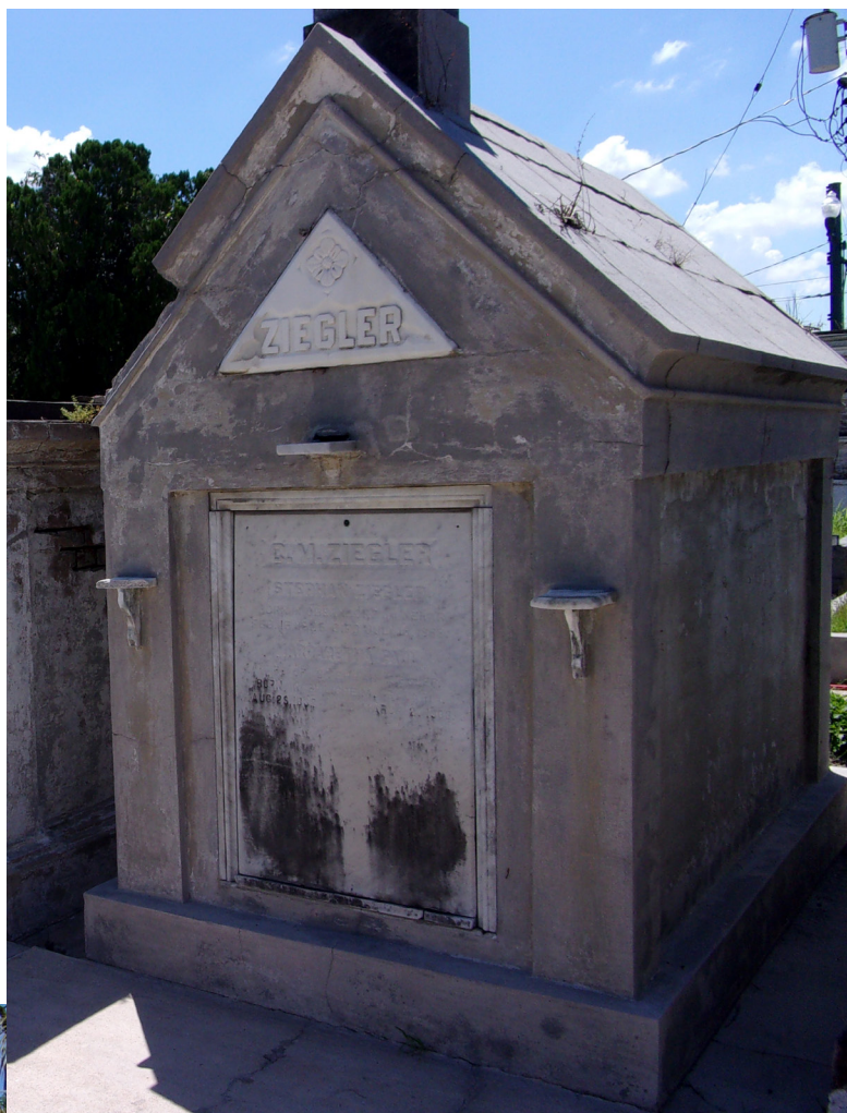
Figure 82 (to the right). Missing portion of pediment, staining and spalling of substrate, and some biological growth out of the roof.
