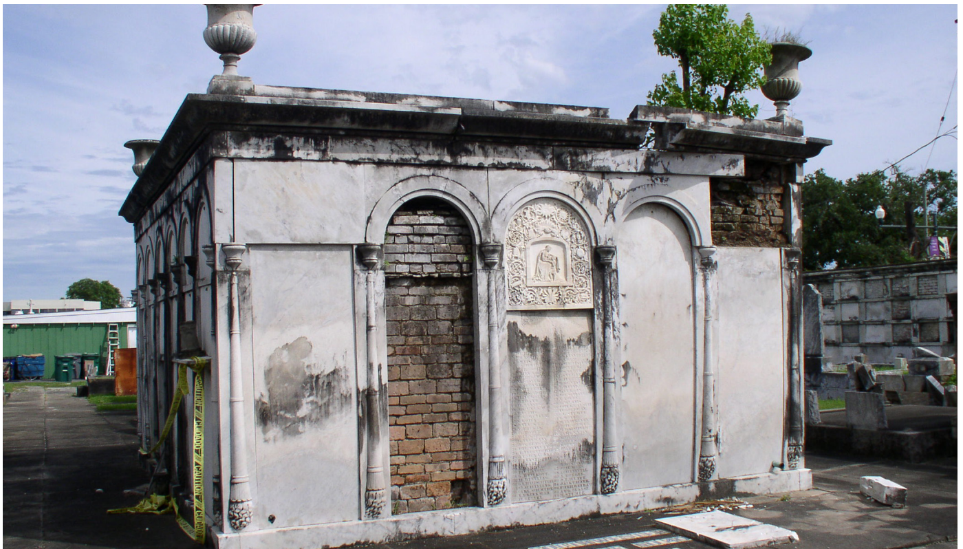
Figure 22. Northwestern facade pre-stabilization, showing the tree growing out of the southern corner of the wall. Taken by Michael Duplantier Sr., 2015.
