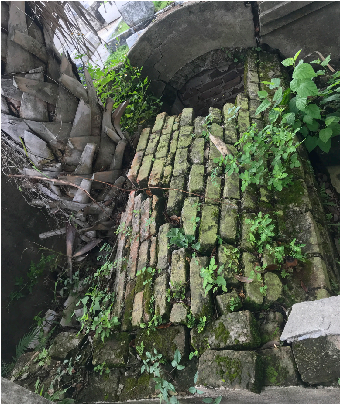
Figure 48. View from rear of barrel vaulted tomb, showing palm tree growth and conditions of the vault.
