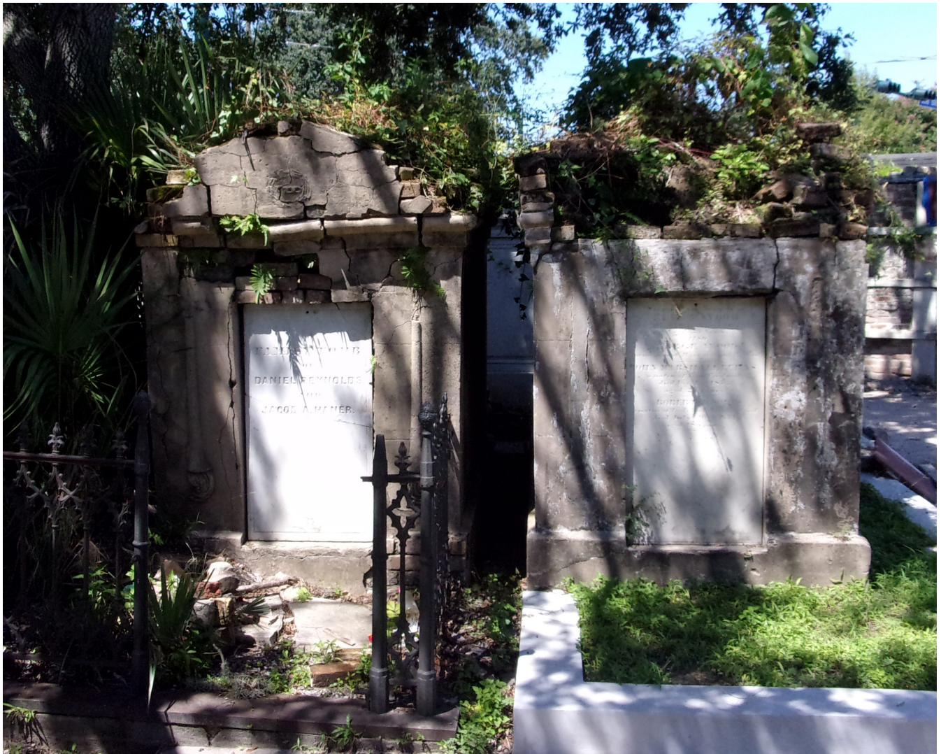
Figure 33. Two tombs in OFR, both in poor condition with crumbling brick walls and biological growth from the roofs.
