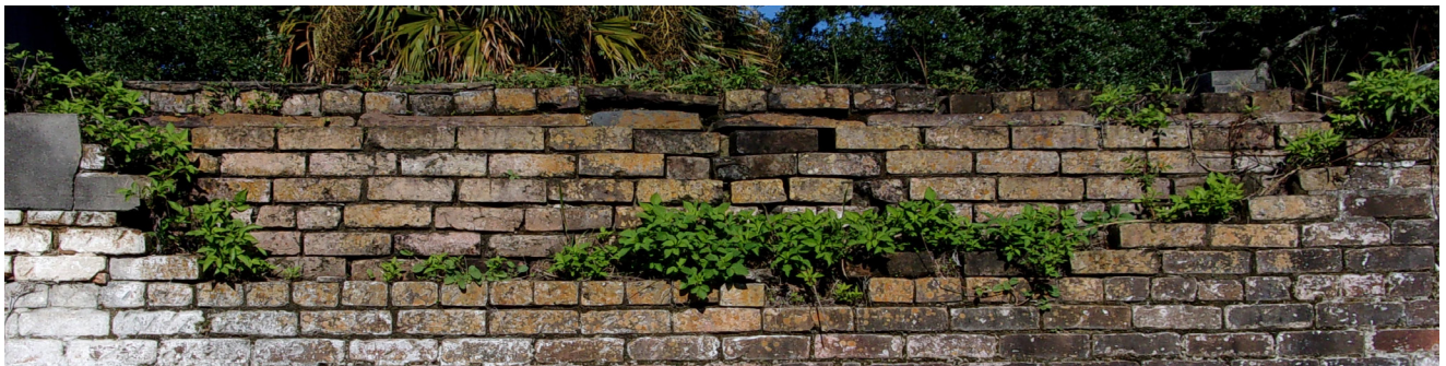
Figure 80 (top). Society tomb showing major crackining and staining and missing closure tablets.
