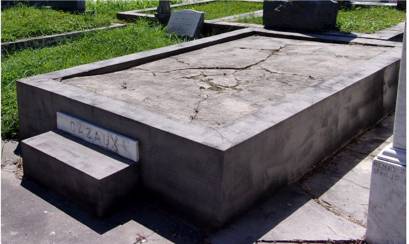
Figure 73. Coping grave, showing relatively good/fair conditions with cracking on the top of the grave.
