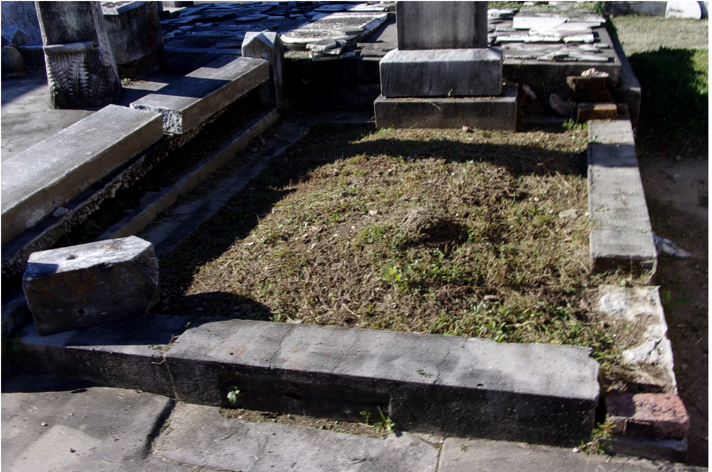
Figure 89. Coping grave in poor condition with cracking and some missing material.
