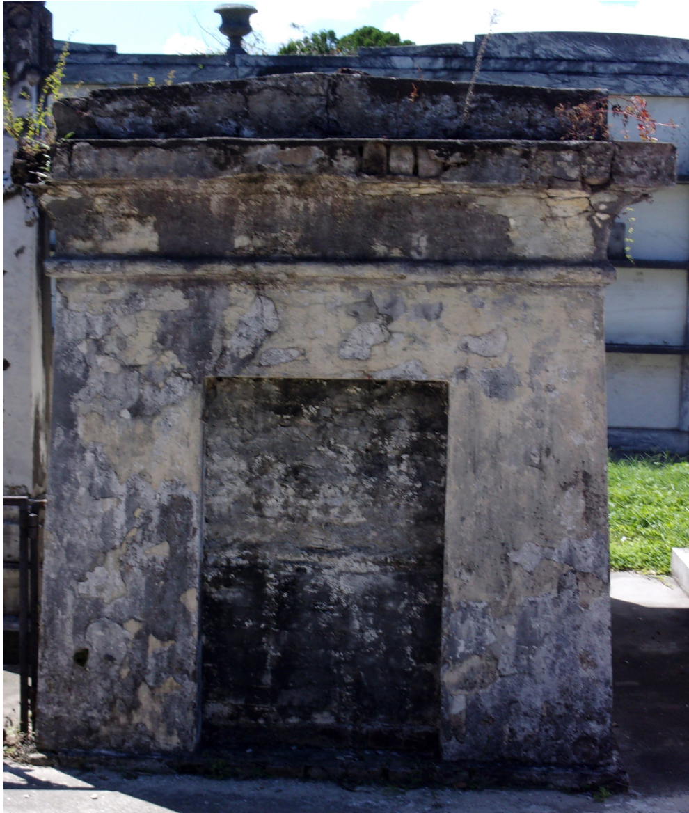
Figure 77. Mostly structurally sound tomb with noticeable biological growth, cracking, and spalling of the stuccoed exterior. Missing closure tablet.
